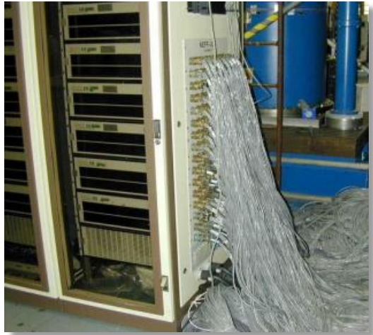
Cabling & instrumentation for 400 wired strain sensors
